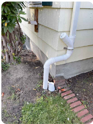
ELBOW FITTINGS AND CAPPED DOWNSPOUT AT EXISTING DOWNSPOUT
