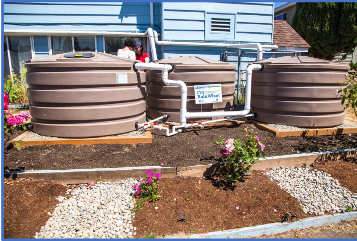
Three 660-gallon cisterns capturing 2,779 square feet of roof area are located in the back of the building, with two overflows to existing catch basins in the parking lot.
